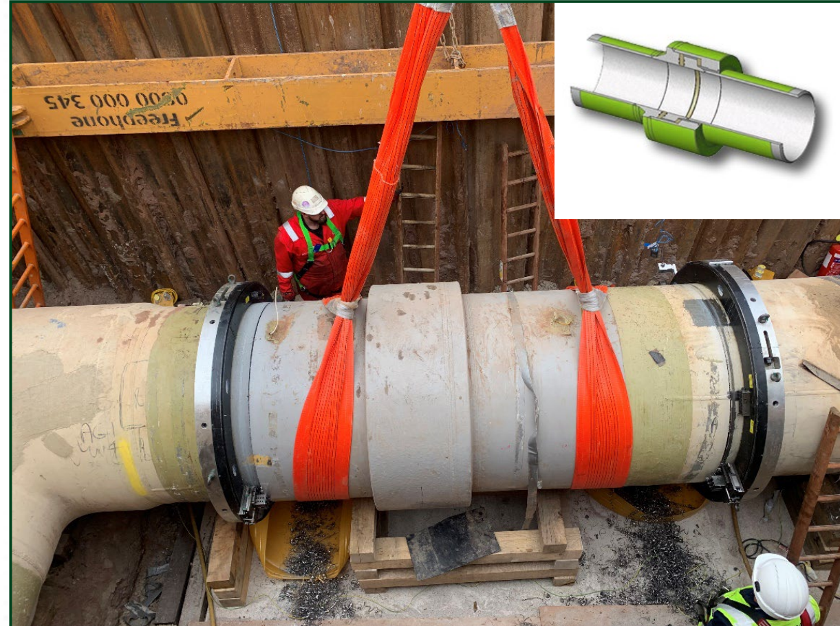
48" IJ – National Gas site - Lochside Multijunction
